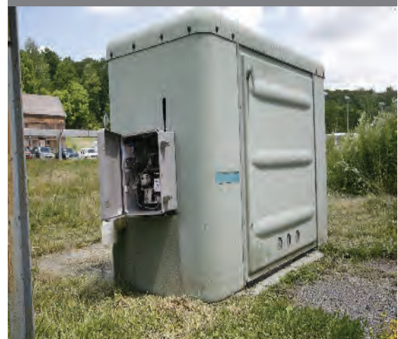
RS-3314 Monitoring Lift Station
