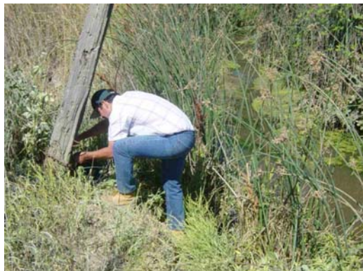
Figure 1. Installing a Telog PR-31 data collector at a spill site.
