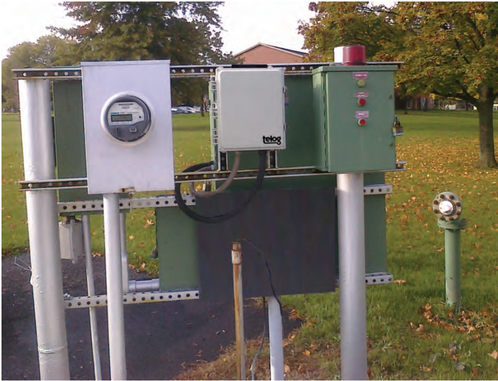
RS-33u monitoring a lift station
